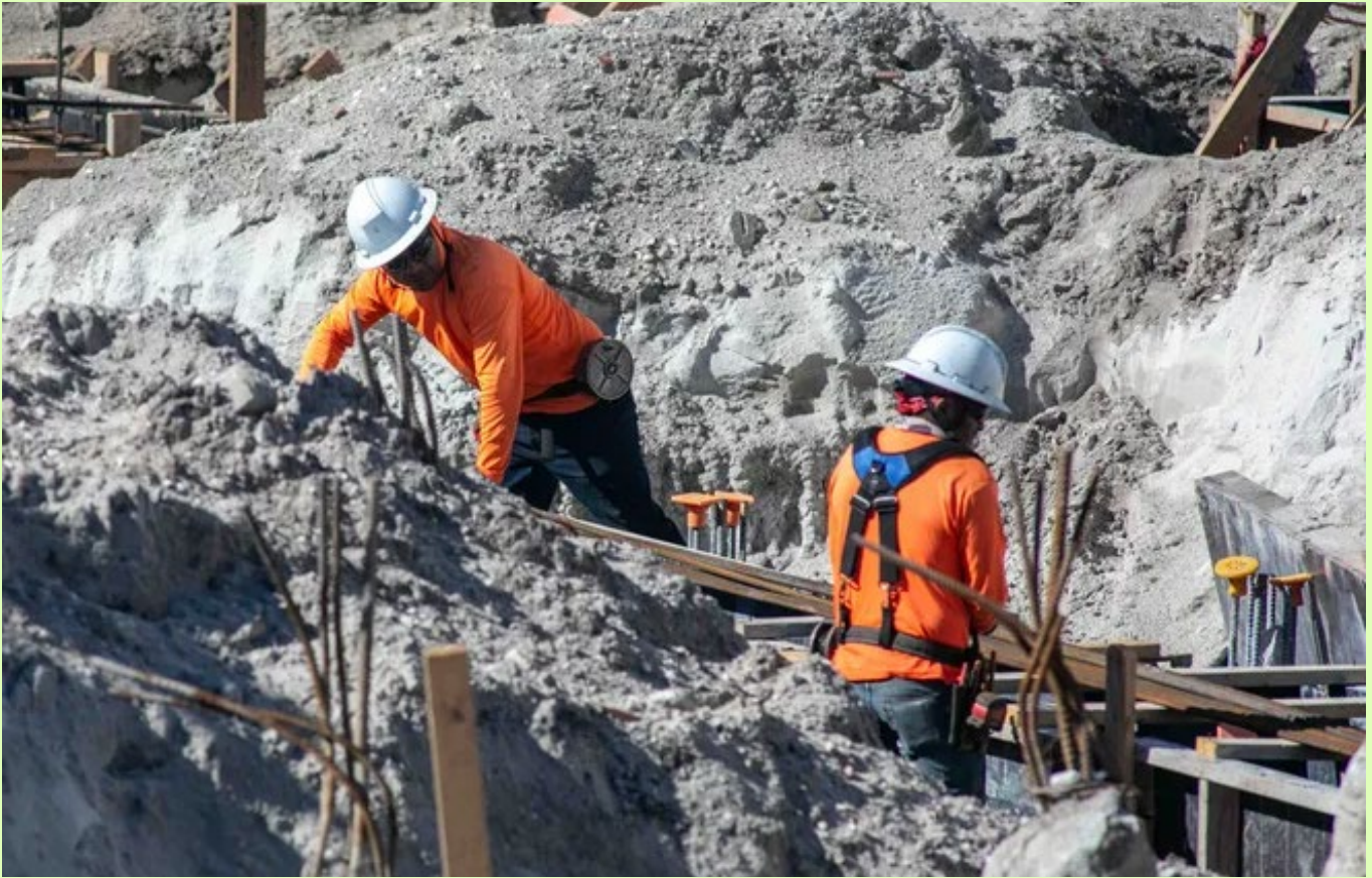
Construction crews, seen on April 5, are working to complete the Royal Poinciana Playhouse's shell structure, including masonry walls, concrete beams, columns, and the rest of the structural steel. [DAMON HIGGINS/THE PALM BEACH DAILY NEWS]
