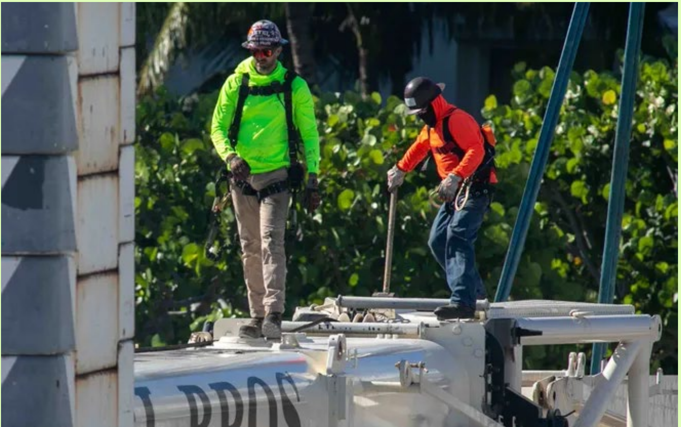
Workers make their way across a large crane at the Royal Poinciana Playhouse construction site April 5. [DAMON HIGGINS/ THE PALM BEACH DAILY NEWS]
