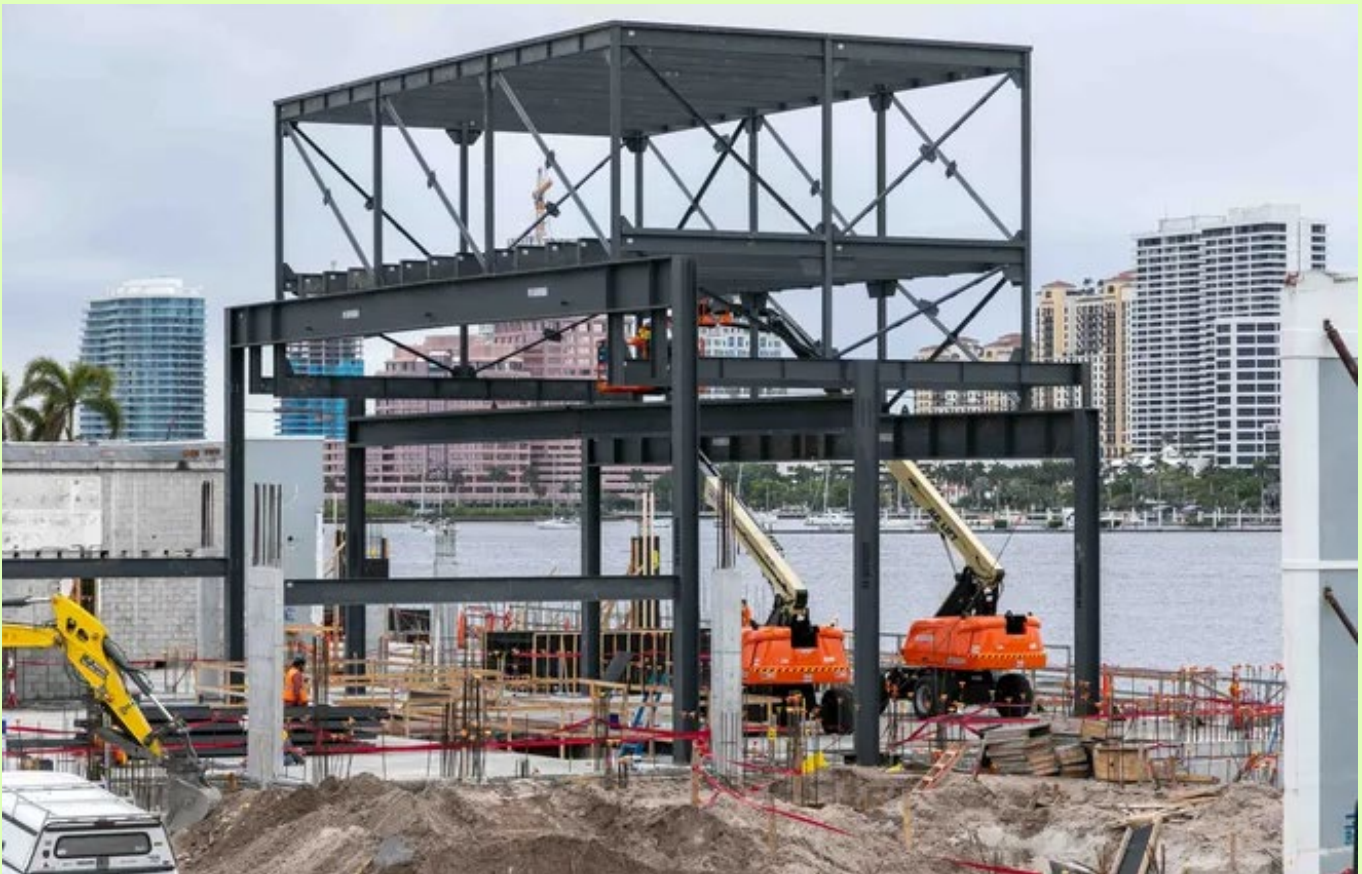
Workers have begun erecting the framework for a multilevel structure at the Royal Poinciana Playhouse construction site on April 4. [DAMON HIGGINS/THE PALM BEACH DAILY NEWS]
