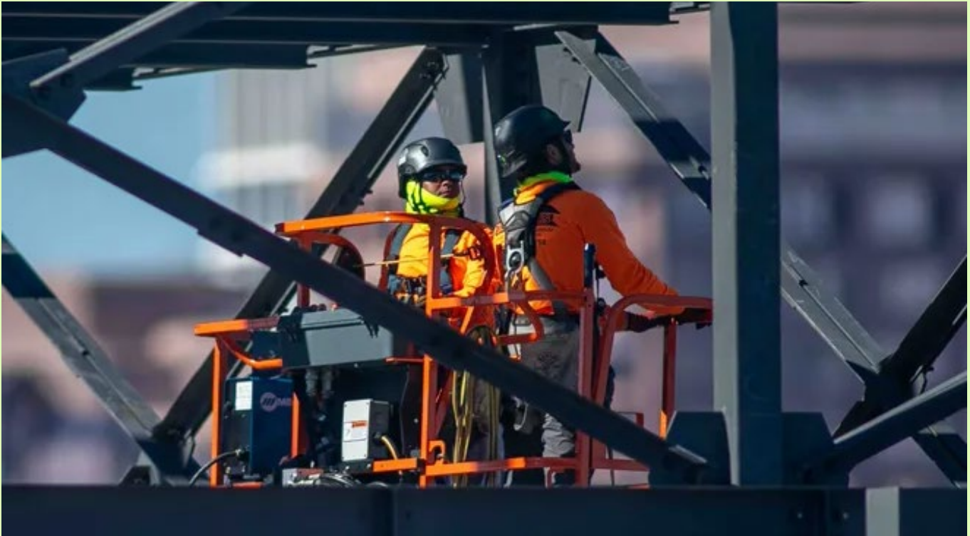
Workers use a lift to help erect a multilevel structure at the Royal Poinciana Playhouse construction site on April 5. [DAMON HIGGINS/THE PALM BEACH DAILY NEWS]
